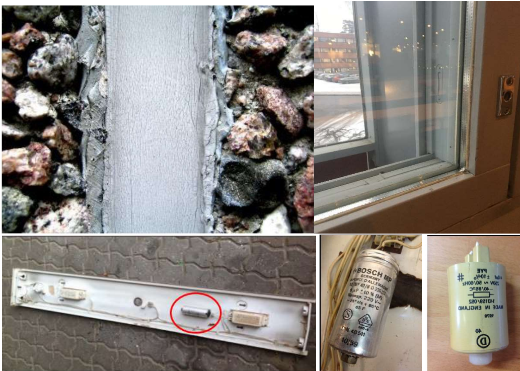
Figure 4. PCB containing sealants. PCB containing condensers in lamps (marked with red circle) and examples of condensers with manufacturing year visible. Photos: Jarno Komulainen, Vahanen Building Physics Ltd (upper left), VTT OY (upper left) & Danish EPA report Miljostyrelsen nr 10, 201518 (photos below)
